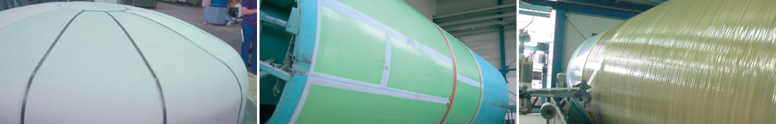
From left to right: Manufacture of the domed base in segmented design; cylinder made of welded SIMONA® PVDF-GK sheets; winding of the cylinder onto the winding mandrel with GFRP
