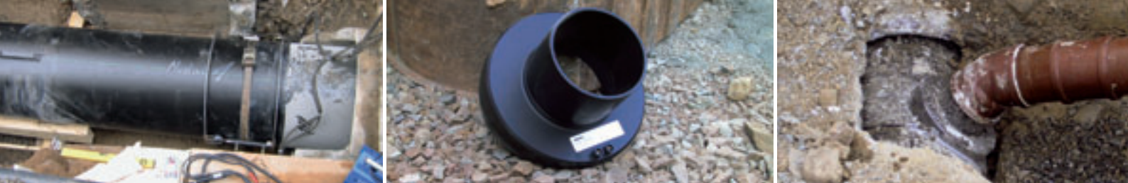
Figs. (from left to right): Welding and feed-in of SIMONA® PE 100 pipe modules SIMOFUSE®, PE 80 external saddle SIMOFUSE® for service pipe connection welded with PE 100 waste-water pipe
