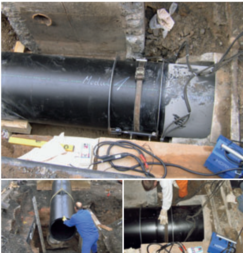
Repair of a defective reinforced concrete pipeline with SIMONA® PE 100 pipe modules SIMOFUSE®. Top: Welding the pipe modules by means of electrofusion welding. Bottom: Introduction of the pipe modules into the excavation pit and the old pipe.
