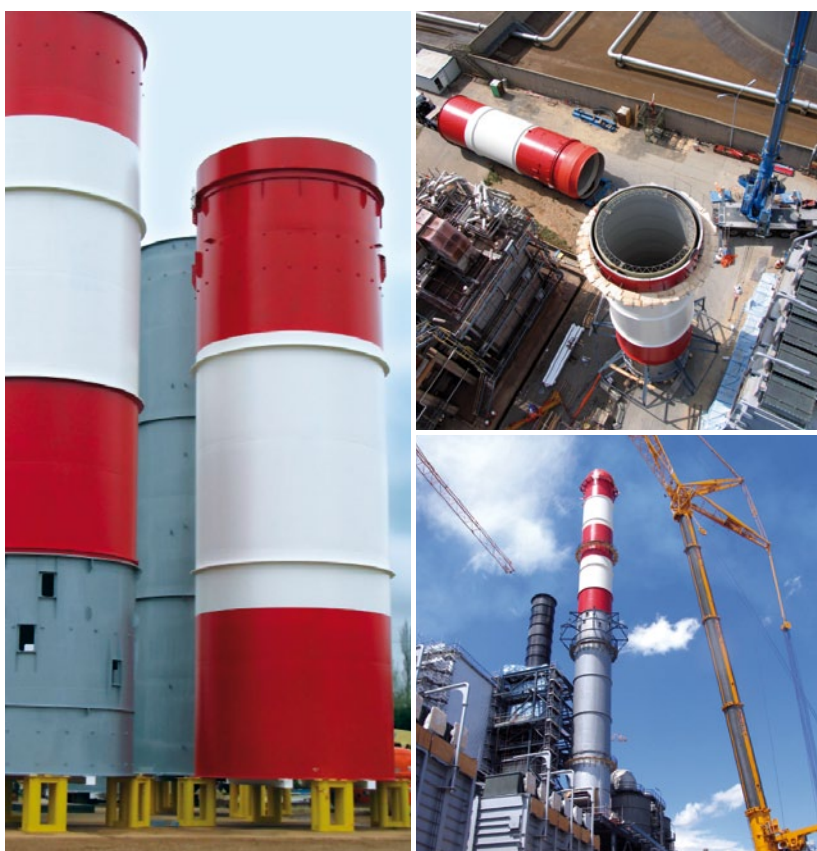
Left: SIMONA® E-CTFE-GK/GRP/steel in-situ. Top right: Before assembly of the last part of the chimney. Bottom right: Completely assembled chimney
