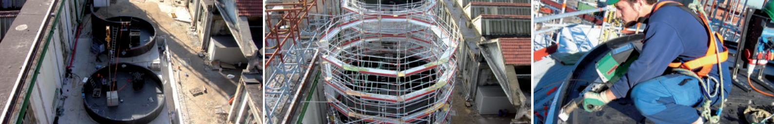
Fig. From left to right: Start of construction, advanced construction section, connection of roof and wall elements
