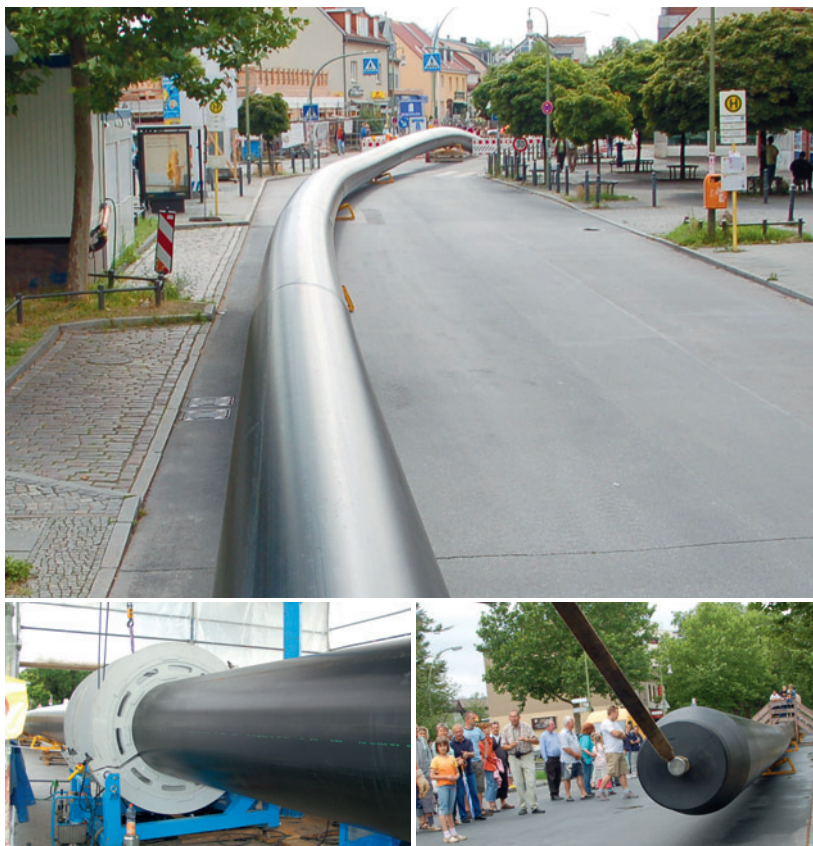
Top: The 500 m long pipeline was drawn into the old pipe in a single feed. Bottom left: The pipelines were welded together by means of heated-tool butt welding. Bottom right: The entire pipeline was transported to the access trench with light construction equipment.
