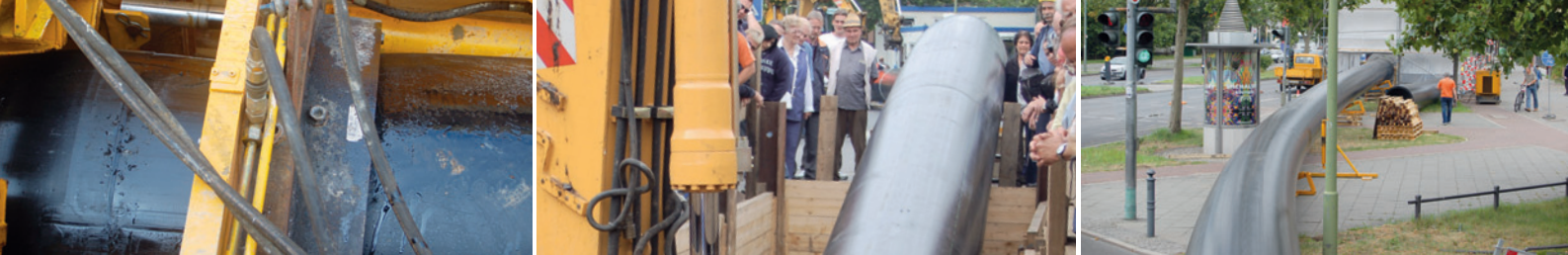
Fig. from left to right: The reducing tool brought down the circumference of the SIMONA® PE 100 pipe from 1060 mm to approx. 970 mm. Small access and exit trenches guarantee minimal disturbance for residents and traffic. The high flexibility of the SIMONA® PE 100 pipes also enabled narrow curve radii.
