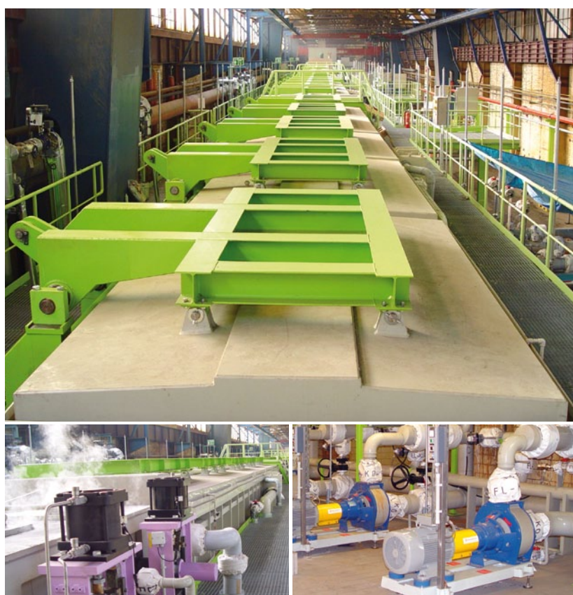
General view of the pickling line and the various tanks
