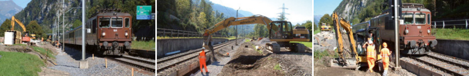
From left to right: Site installations and pipe storage area next to the railway line in service; standard-compliant pipelaying in the drain trench; confined space and full railway service during the construction phase called for maximum reliability and precision
