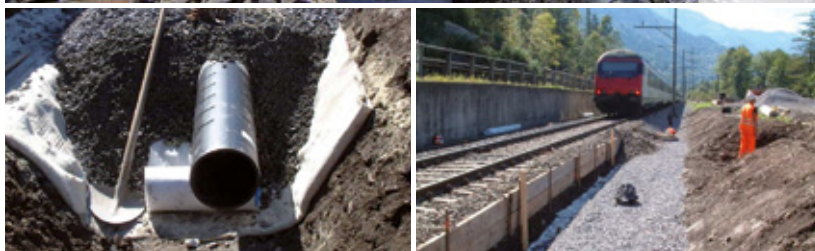
Top: Open drainage trench with 2/3 slotted SIMODRAIN® pipe, next to the railway line; Bottom: Geotextile jacket for the filter gravel bed
