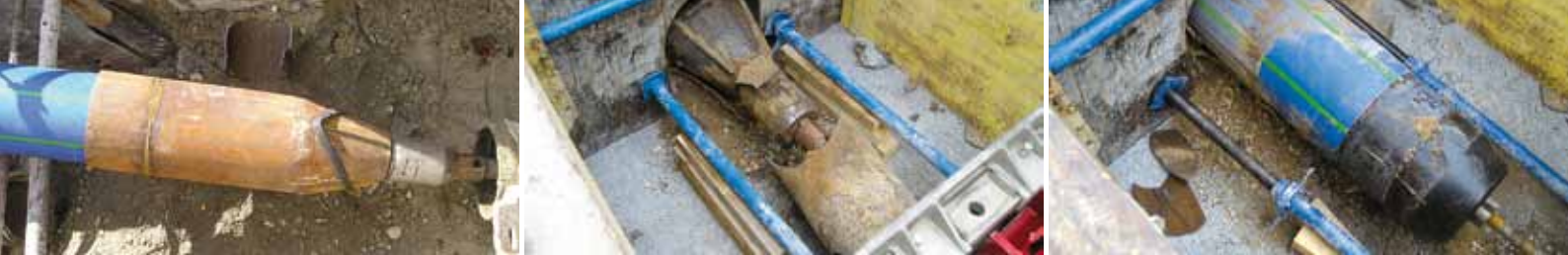
From left to right: the bursting head, including a new SIMONA® SPC RC drinking water pipe, is inserted into the old pipe. During insertion it destroys the old pipe, displacing it into the surrounding soil, and the drinking water pipe finally arrives in the destination pit.
