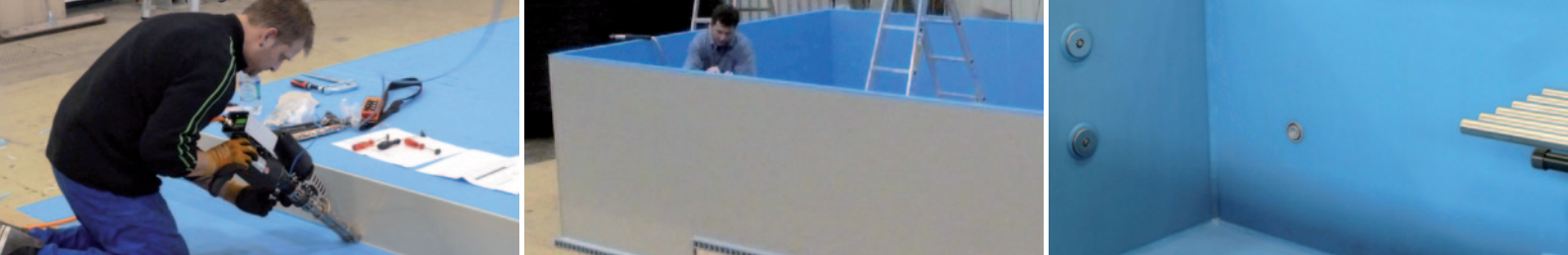
From left to right: fitting the stepped bottom; fastening the side walls; installing the nozzles, spotlights and valves
