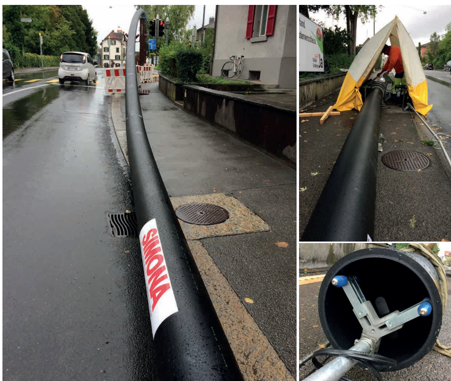
Left: the pre-welded SIMONA® PE 100 Liner Pipe string; top right: welding (heated-tool butt welding) of the SIMONA® PE 100 Liner Pipes; bottom right: after welding both the internal and external beads are removed with a special-purpose tool
