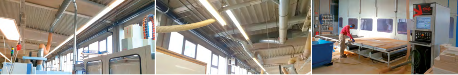
From left to right: The SIMONA® PE 100 Pipes and Fittings are installed along the entire ceiling of the building. An employee in front of the company's largest CNC milling line.
